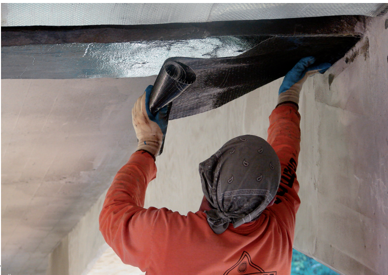
Jericho Bridge - Ohio USA stage of work Jericho Bridge - Ohio USA fase di lavoro
